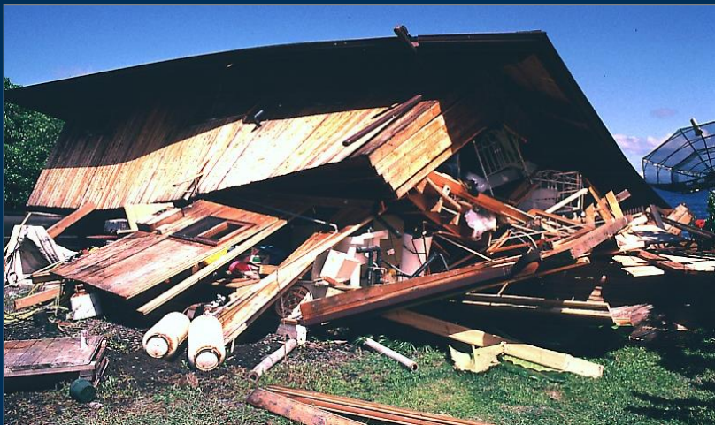
Collapsed home in Kalapana, Hawai'i. USGS photo.
