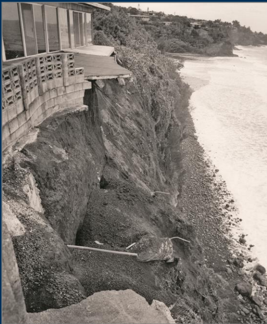
Coastal damage on the Island of Hawai'i. Photo by Larry Kadooka, Hawai'i Tribune-Herald.
