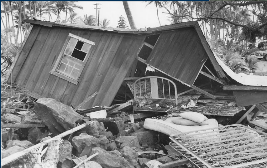
A Punalu`u house demolished by the 1975 tsunami. Photo by David Shapiro, Honolulu Star-Bulletin.
